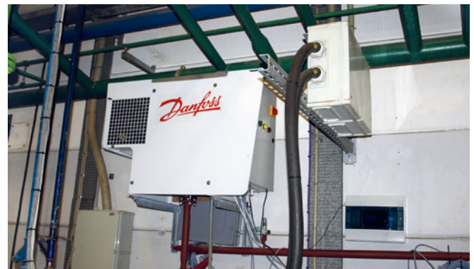
Danfoss IPS installed at Agri-Norcold plant, Kolding.
